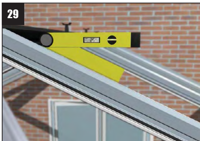
Check that the pitch of the roof is correct. Your Surveyor should have provided a drawing/a copy of the roof confirmation which displays the pitch.
