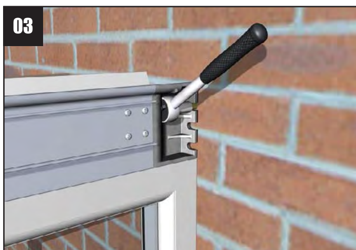
Where the eaves beam sits against the host masonry wall, it has a structural moulding attached to the eaves beam. This has three fixing positions cast into it to allow attachment into masonry – choose the hole that directly lines up with solid masonry and drill a 10mm hole into the host wall. Attach the structural moulding using the M8x80mm anchor supplied. Silicone seal the gap where the moulding attaches to the eaves beam.
