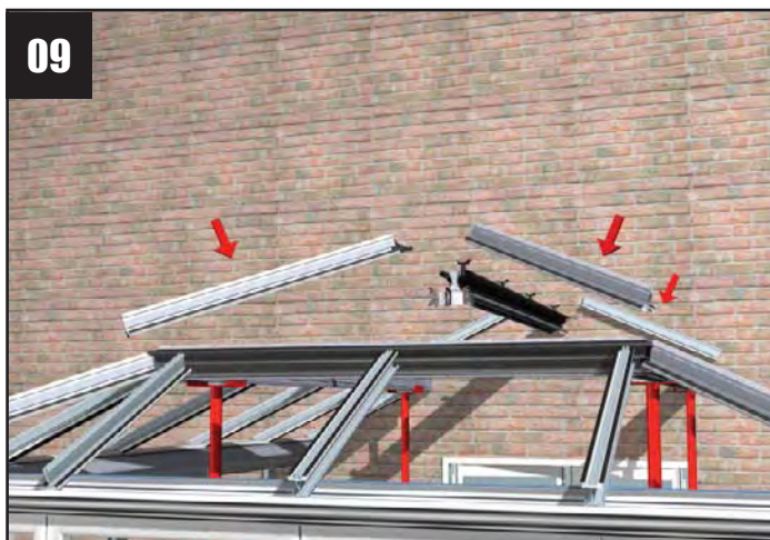
Using the roof location plan, build the upper roof as per section 5 of this guide
