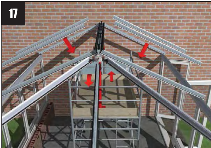
17 Continue to attach all the glazing bars using the location plan provided to check each bars final position with its corresponding label.
