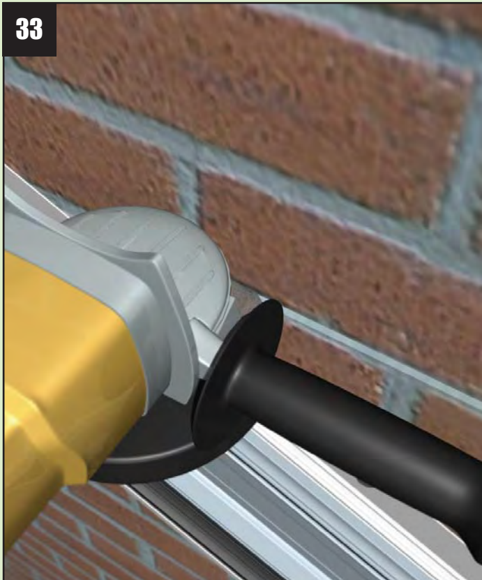
33 Ensure the pre-formed soaker is clipped into the starter bar. At this stage it is easiest to mark and cut out for the lead flashing. For best results always grind a 35mm deep slot to allow Conservaflash to be let into the wall. Brush out any dust from the channel.
